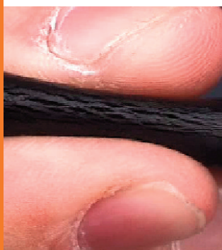
By pinching the liner stem, it is easy to see the small cracks that appear as the liner ages and deteriorates.
